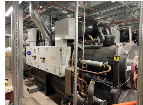
Figure 2.7: Citigen network energy centre plant – heat pump.
